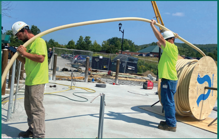
Oxygen main line for medical center.
