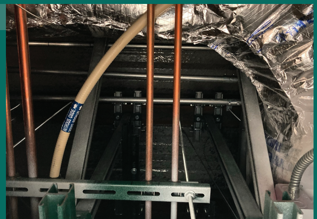
MediTrac® installed above a finished operating room ceiling.
